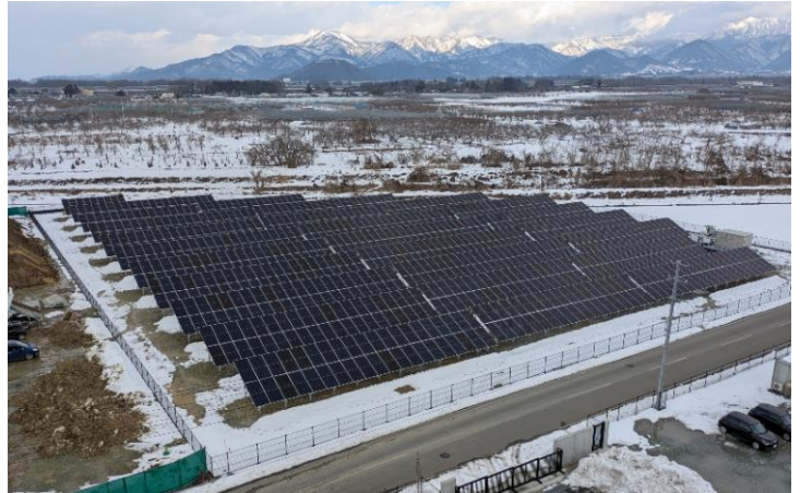
<Tendo Factory: 700kW PPA-Based Power Generation Facility>
